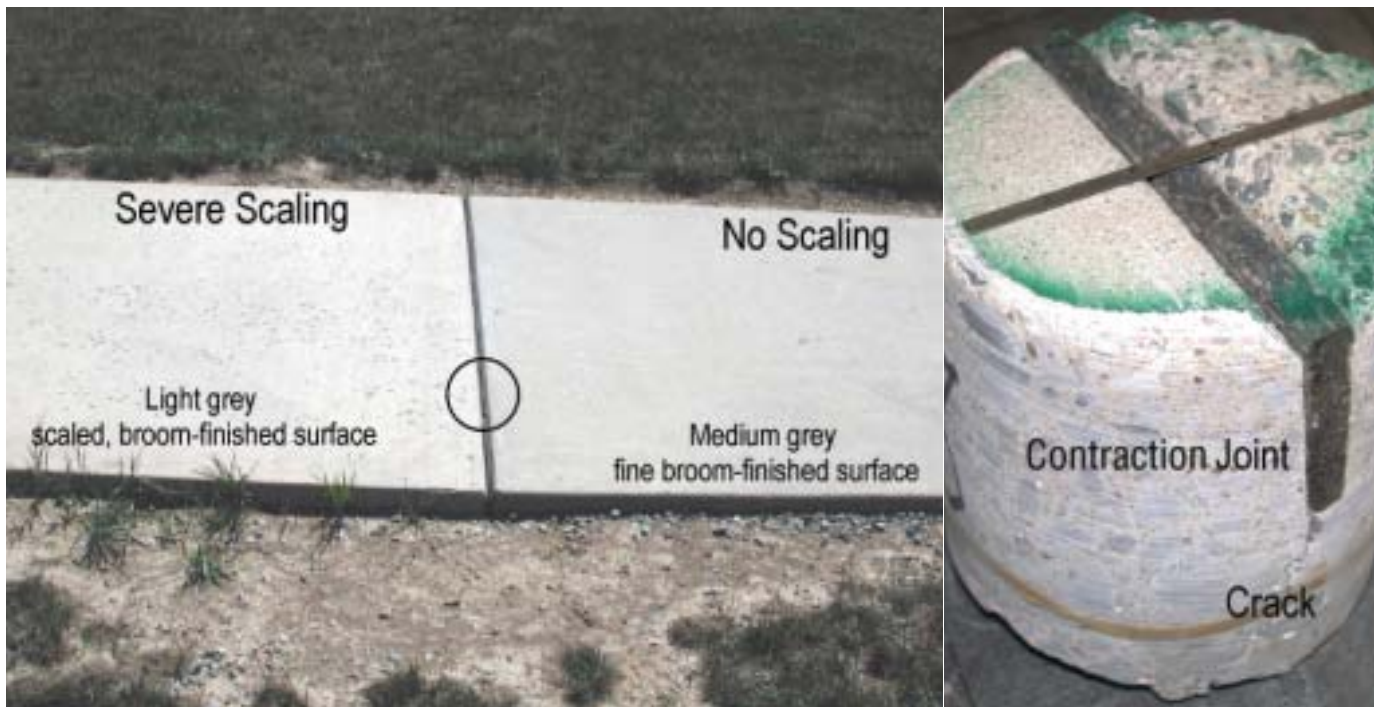
Fig. 2: Case study II (Scaling due to finishing in the presence of excess water at the surface)—Concrete core from a contraction joint showing adjacent sound and scaled surfaces
