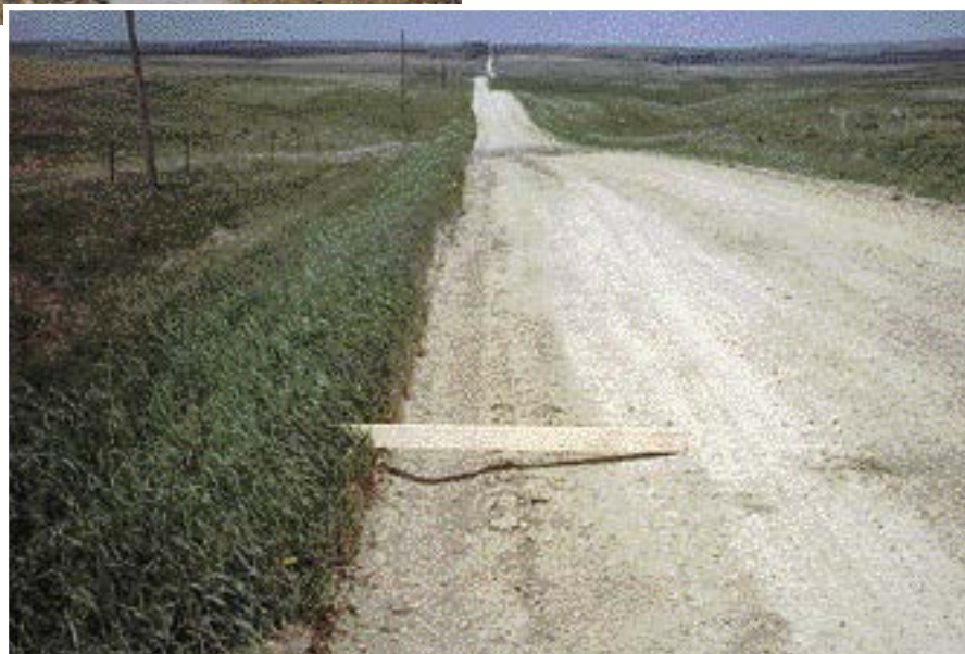
Secondary ditch over six inches deep.
