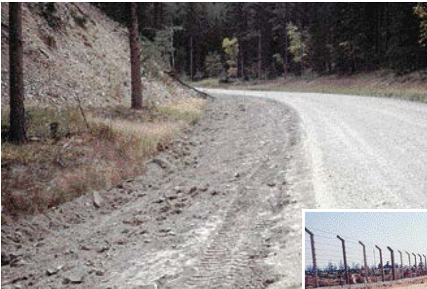
A nicely reshaped ditch that meets the shoulder line of the road and allows good drainage.
