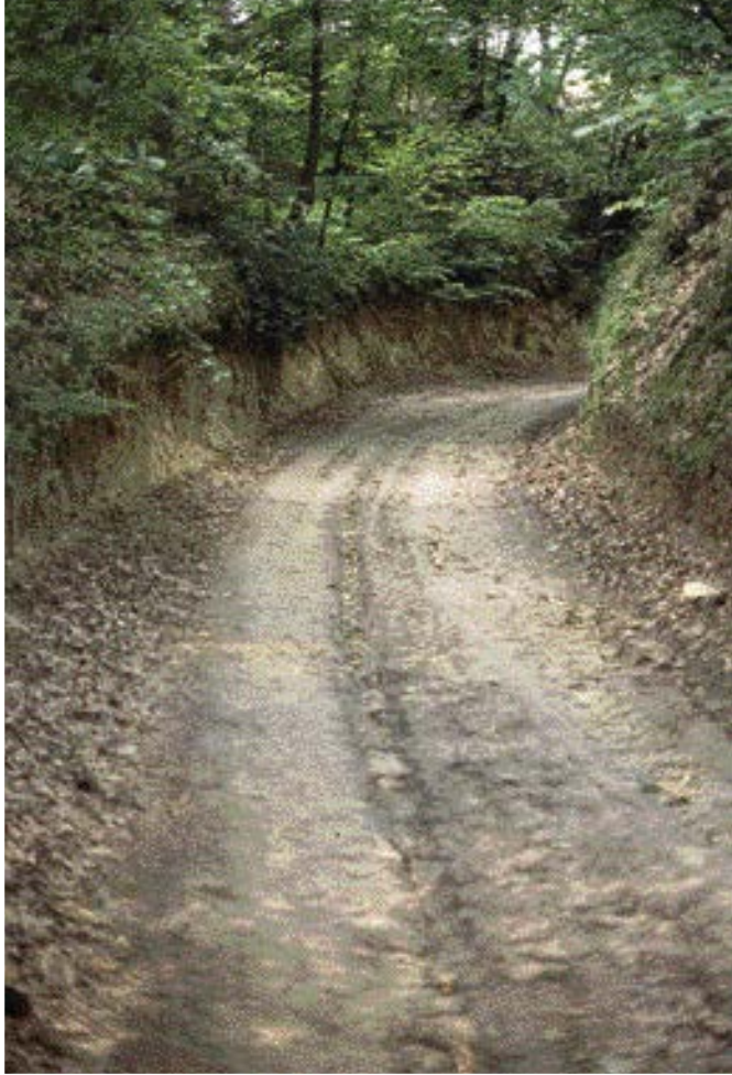
This road, located in Poland, has very poor cross section with no ditches. Consequently, water drains down the roadway itself and after many years of erosion, the roadway is several feet lower than its original elevation. (Courtesy of Mary O'Neill, Office of Remote Sensing, South Dakota State University)
