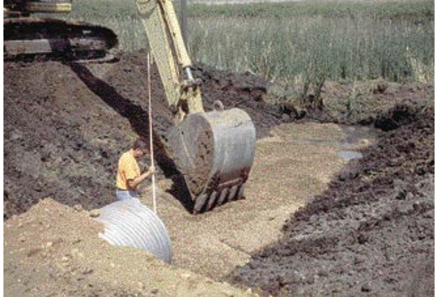
New culverts installed well and at correct elevation are essential for carrying water under a road. A reasonable maintenance schedule is required to keep them functioning well.
