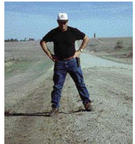
The windrowed gravel is then brought back over the recovered material and the roadway is restored to proper crown and shape. The high shoulder has been eliminated.
