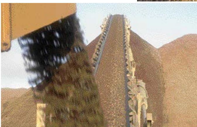
The discharge conveyor from a crushing plant is in the foreground. Notice how badly segregated the material is as it is carried up to the stockpile on a belt stacker. This invariably leads to problems illustrated in the following two photos.
