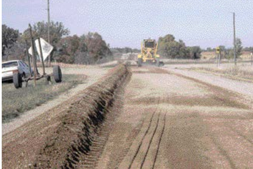
The motorgrader operator has done a good job of picking up the fresh gravel and equalizing it into a very uniform windrow.
