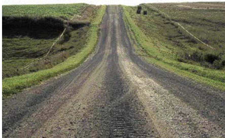
A gravel road with a 26-foot driving surface, yet everyone drives in the middle. The primary reason is excessive crown.
