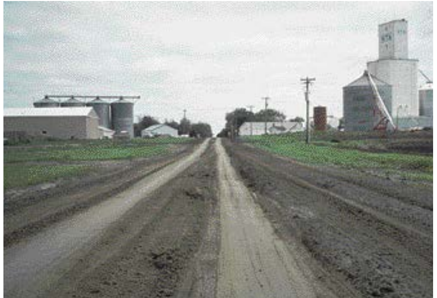
This gravel road shows severe distress after being subjected to a heavy haul from trucks hauling wheat to a grain elevator. The problem was made worse by an unusually wet season.
