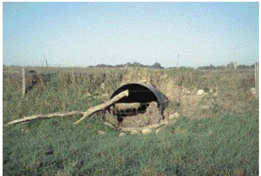
This road could fail if debris is not cleared before the next heavy rain.
