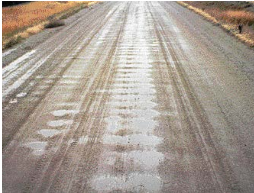
A road that lacks good crown. There is also centerline corrugation (washboarding), a problem that will grow worse when there is inadequate crown.
