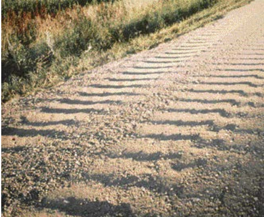
This type of corrugation, "washboarding," is caused by lack of moisture, hard acceleration, aggressive braking, and poor quality gravel.
